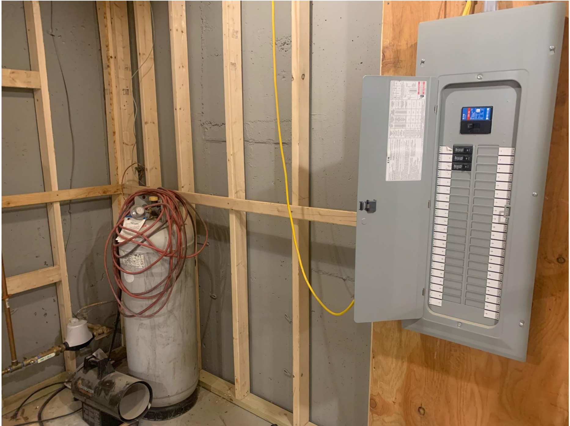
Inside – Level 1 – Garden Level – UUtility Room
