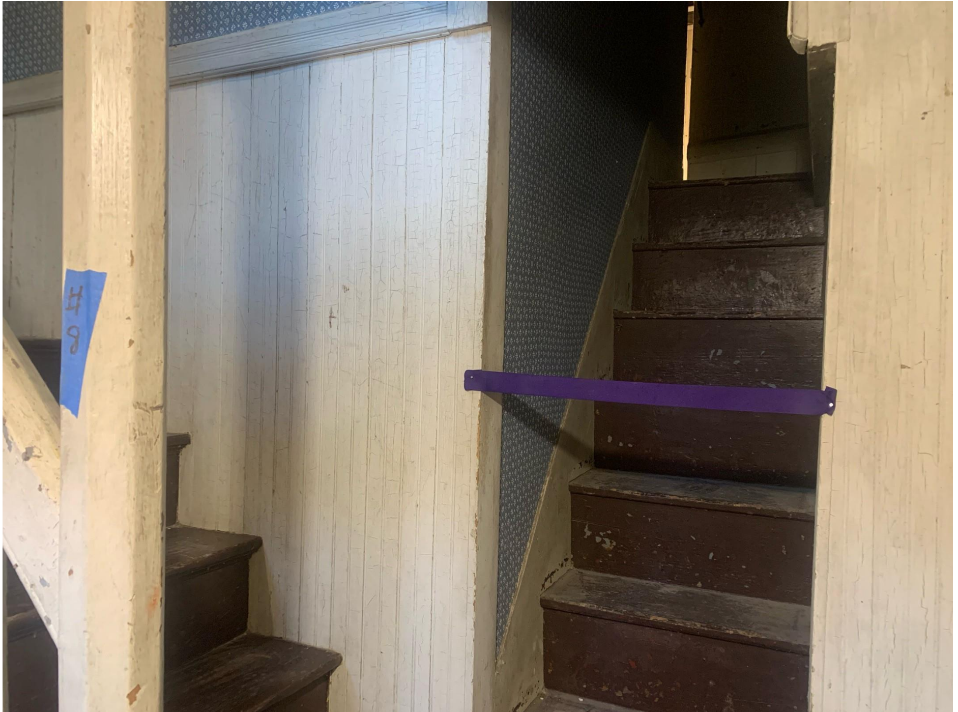
Inside – Level 2 – First Floor – Front Hall – West to East with Back Stairs up to Second Floor
